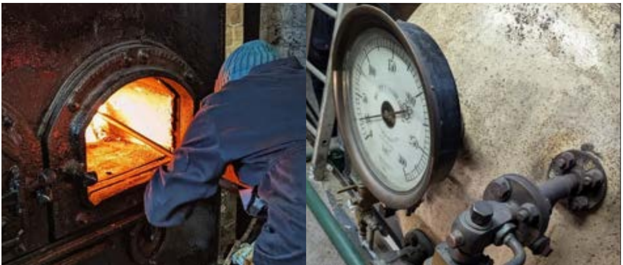
Left: Stoking the boiler. Right: The boiler pressure gauge. Both images: Kieran Gleave
